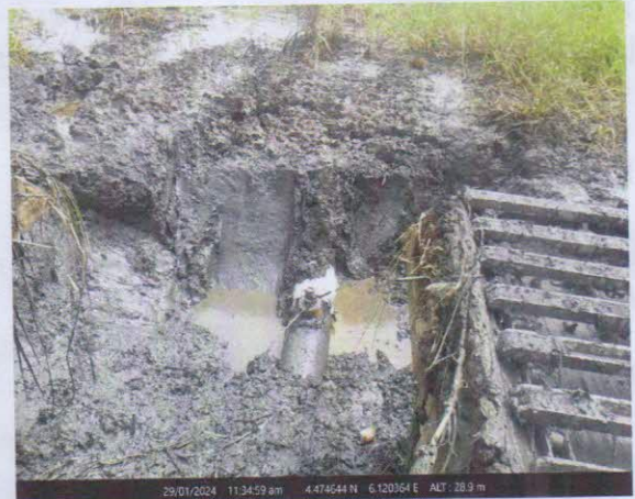
Incident point with 3" Valve Installed
